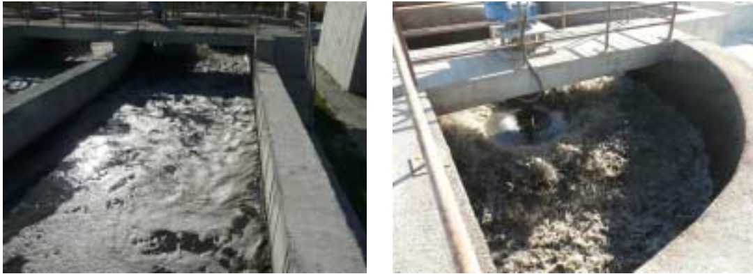
Picture 3.8 Activated sludge tanks + one of the surface aerators
