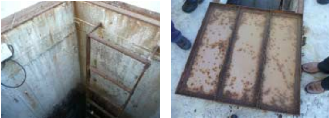
Picture 3.4 Influent receiving basin + cover of influent receiving basin
