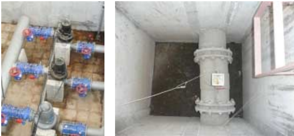
Picture 3.5 Influent pumps in dry well + flowmeter in separate basin
