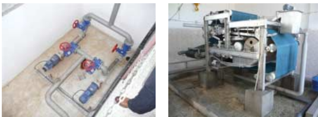
Picture 3.17 Thickened sludge transporting pumps + belt filter press
