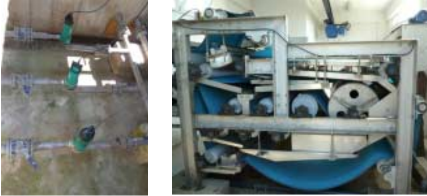
Figure 4.11 The 3 excess sludge pumps + the belt filter press
