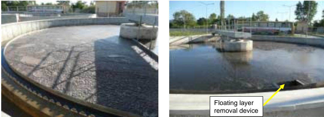
Picture 3.12 Settling tanks
