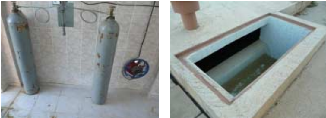
Picture 3.19 Chloric gas bottles + part of chlorination unit
