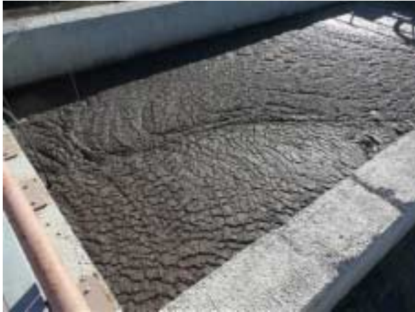
Picture 3.9 Floating layer on activated sludge tanks
