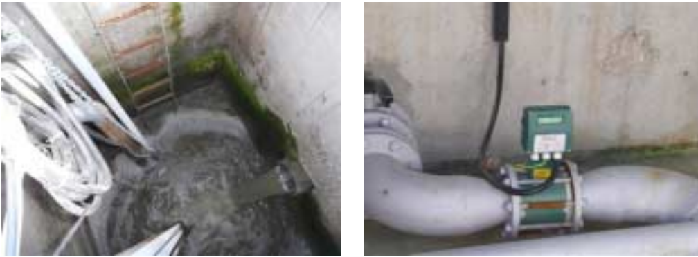
Picture 4.4 Pump basin + flow measurement in dry basin
