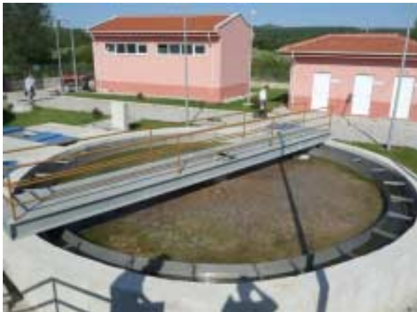
Picture 4.8 One of two settling tanks
