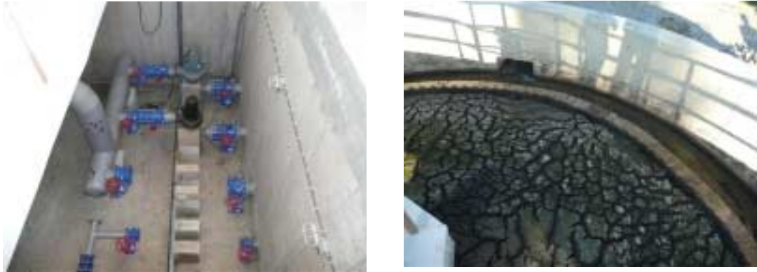
Picture 3.16 Excess sludge pumps + sludge gravity thickener
