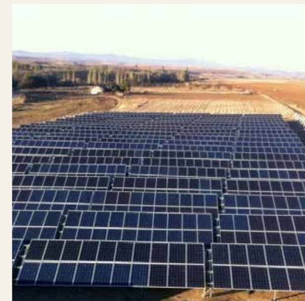
Kırşehir/Kaman, Solar Power Plant
