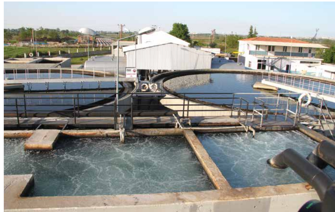
Samsun, Bafra Municipality Potable Water and Treatment Plants
